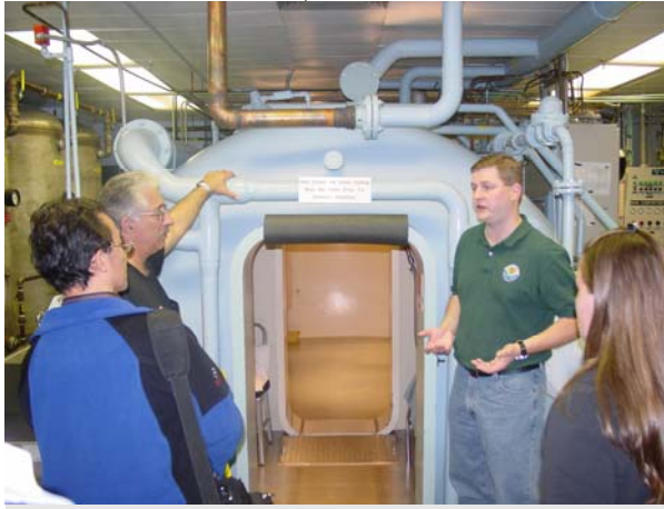
One of Tony's technicians, showing us the entrance to the large chamber.
